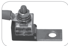
Fig. 7. Fuse MRBF and Positive cable fixed to the CFBAR
