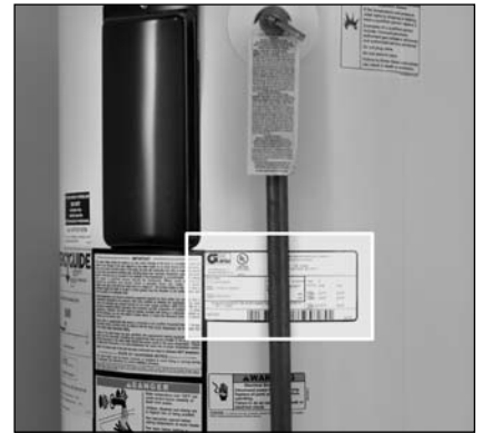
The water heater’s electrical requirements can be determined from the data plate.
