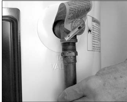
The T&P Relief Valve discharge pipe must be installed properly and piped to an adequate drain.
