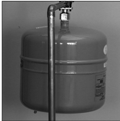
Figure 16 - The Thermal Expansion Tank should be pressurized with air, to match the home's incoming water pressure.
