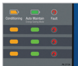
Battery fault detection LEDs
