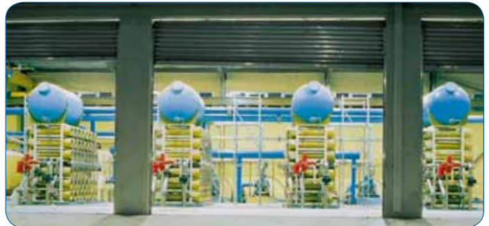
This Culligan Reverse Osmosis Desalination Plant churns out approximately 2.4 million gallons of water per day
